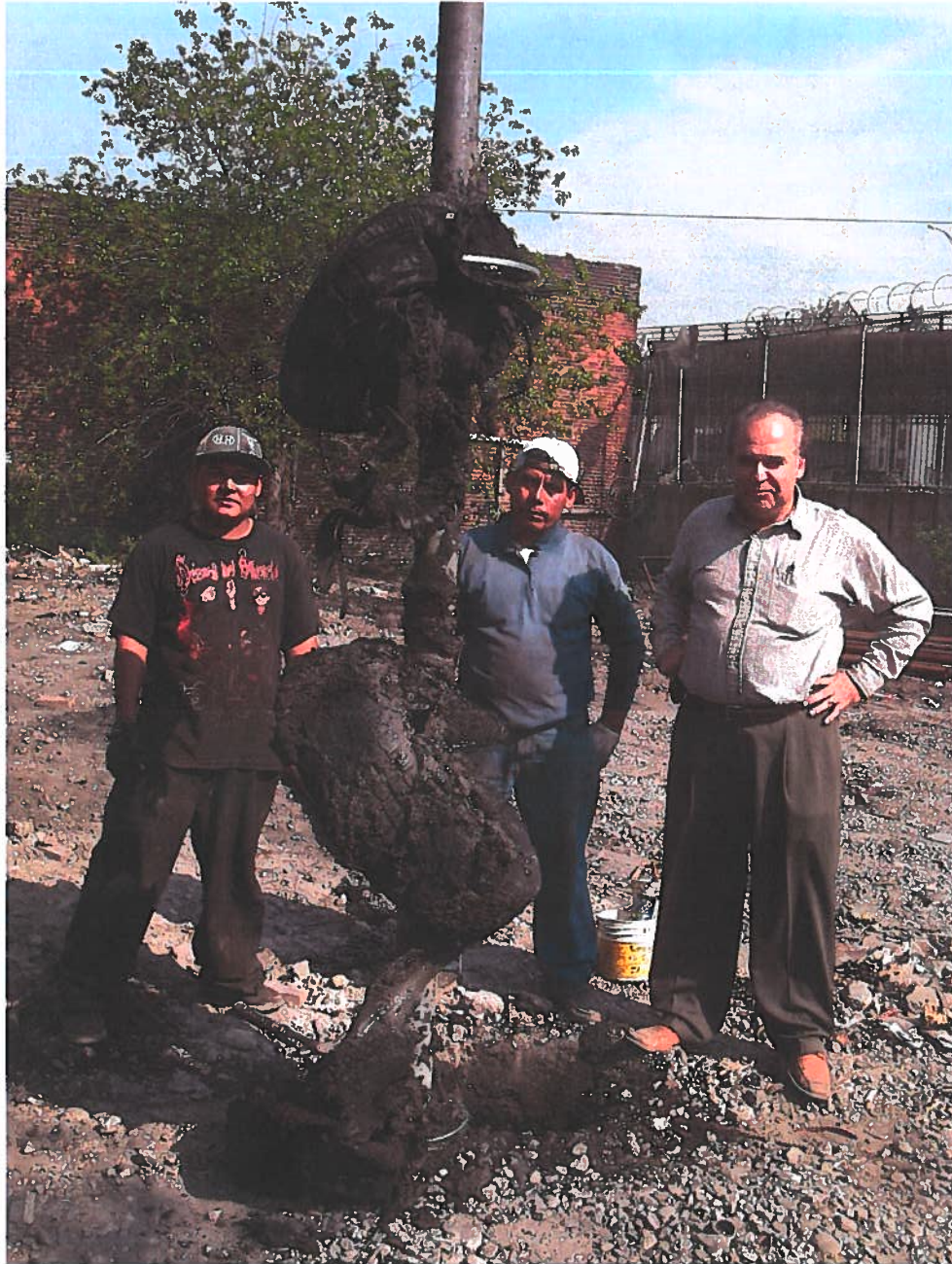
FIG. B-38 Obstruction Encountered in Driving Piles through Backfill.
